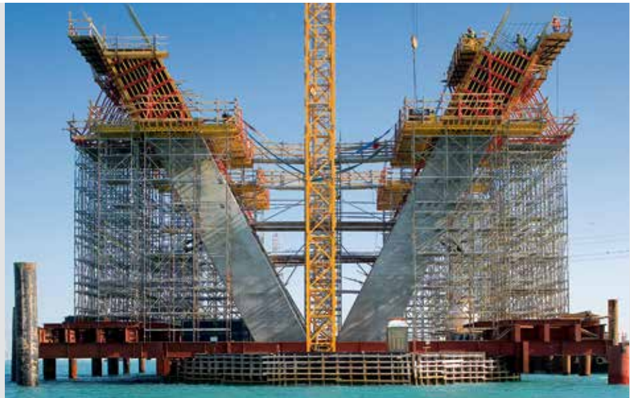
Adaptable trusses for transferring fresh concrete loads and as temporary structure support.
