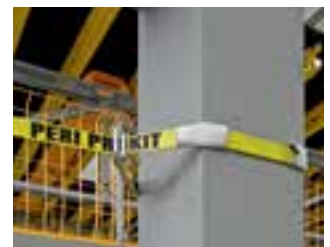
For preventing any damage to the support edges, a plastic hose is used which is pulled over the tension belt.
