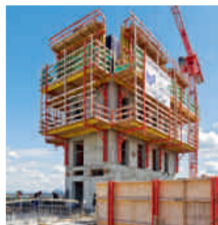
The RCS Rail Climbing System used as formwork scaffold for the building core and as a climbing protection panel on the facade.
