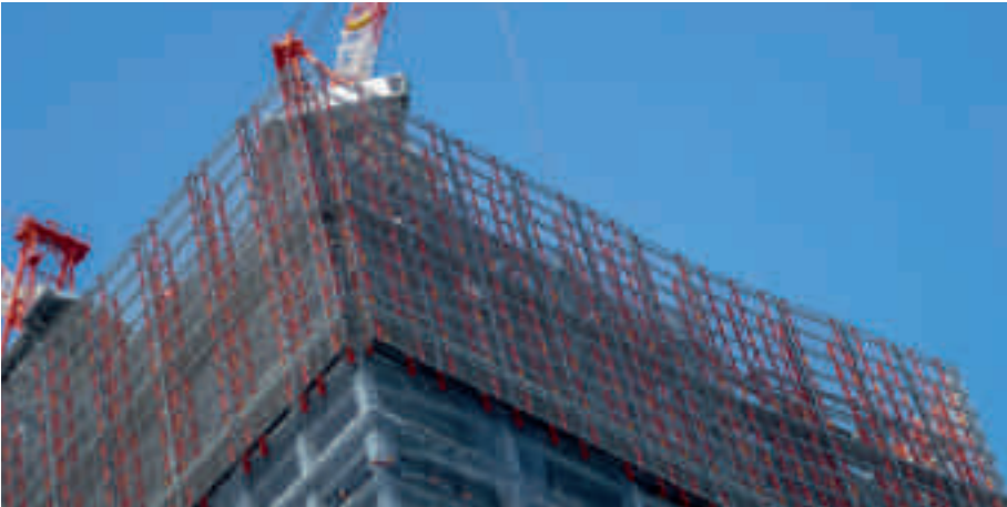
This gap-free mesh enclosure in Japan ensured a high level of safety while simultaneously providing light and air permeability.
