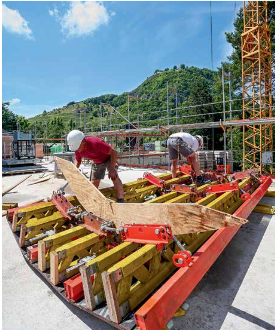
Checking the required curvatures is carried out by placing the radius template on the formwork girders.
