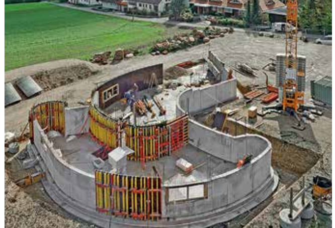
Exceptional challenge in housing construction: reinforced concrete walls with constantly changing radii and offset residential floors.
